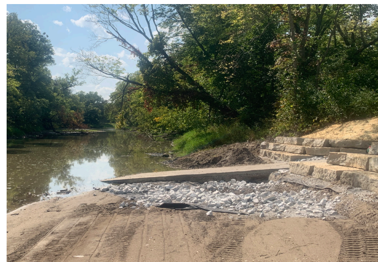
A major improvement paddlers will notice is the new concrete boat ramps providing easier access to the South Skunk River. This view faces downstream from Soper's Mill Access.
