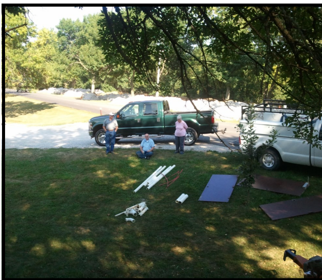
ICCB members and volunteers take a break from assisting with the tear-down of the old showerhouse.
