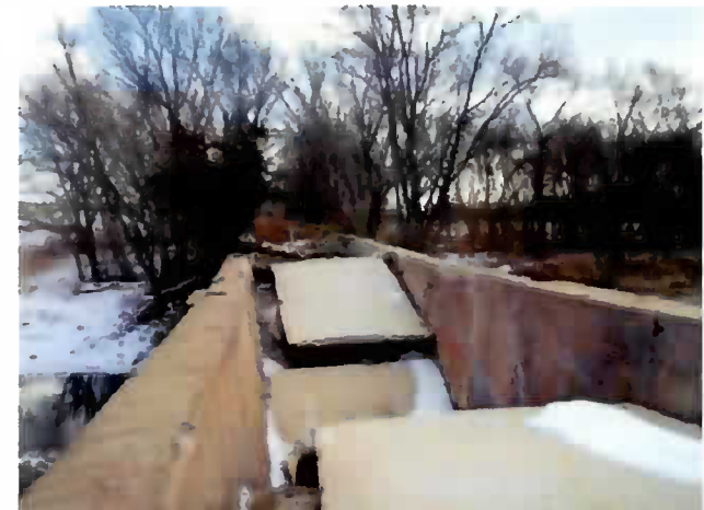
Photo showing McFarlane Bridge deck after the floods of 2008.
