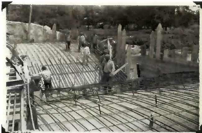
Construction Photo of the Mason City Stewart Ave. Bridge in 1914. Similar Construction as McFarlane Bridge.
